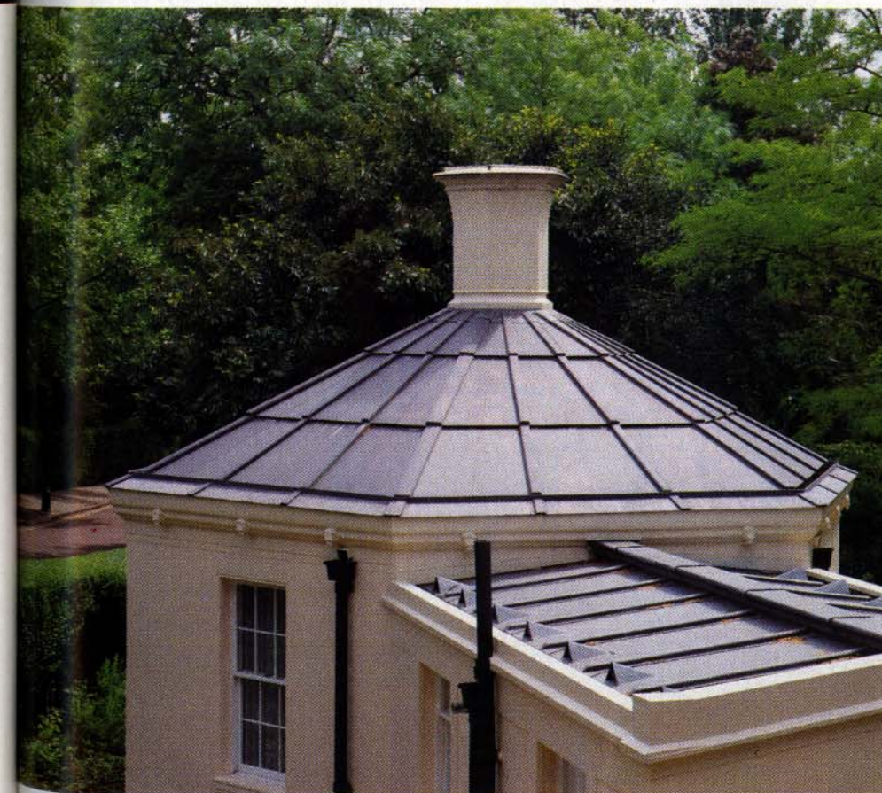
Opposite page: the newly-restored South Lodge. Above: detail of the hexagonal slate roof
