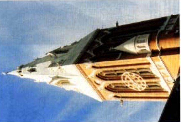
The clock tower - cleaning away the pollution which had given it a dark red appearance revealed the bright red, smoked salmon coloured brick.
